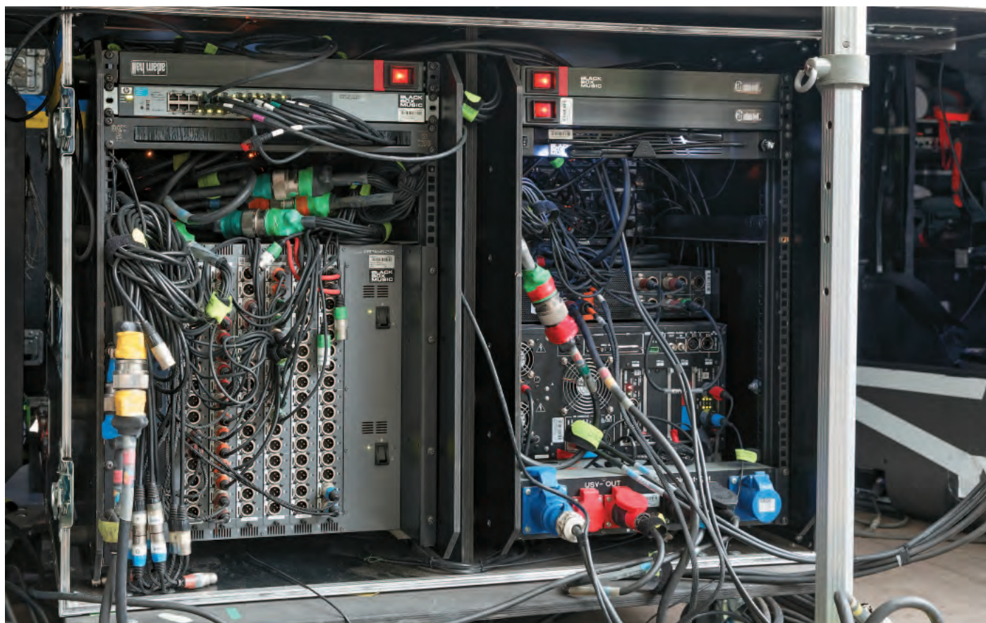
RPio622 I/O rack for the outputs under the monitor console
